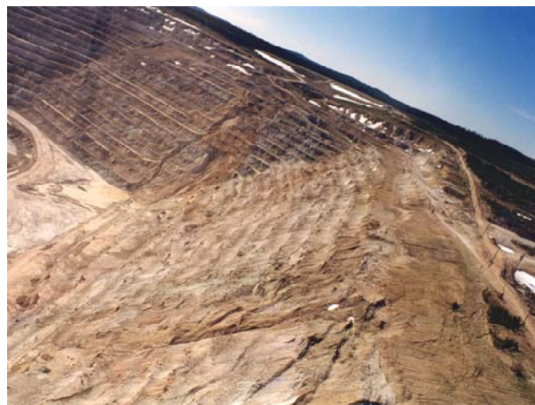
Figure 1- Tension Cracks in Upper Slope of Highland Valley Copper's Lornex Southwest Wall
