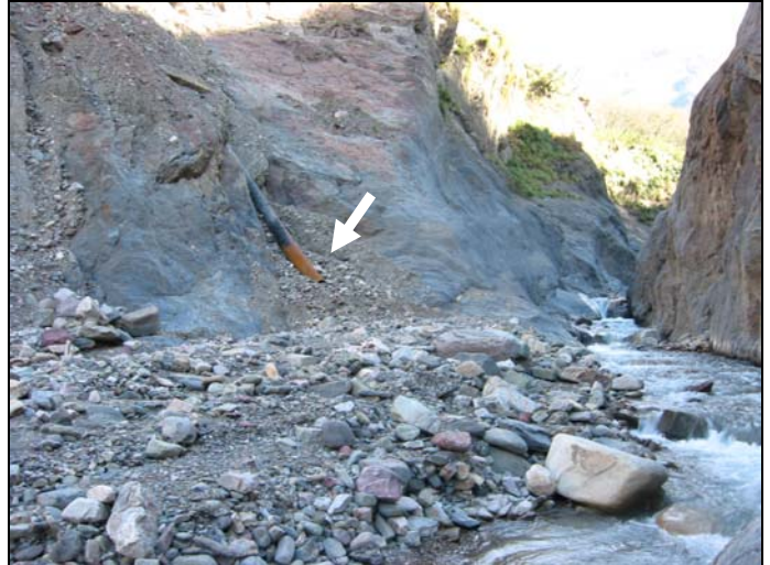
Figure 2. Looking Upstream at the Failed Crossing
