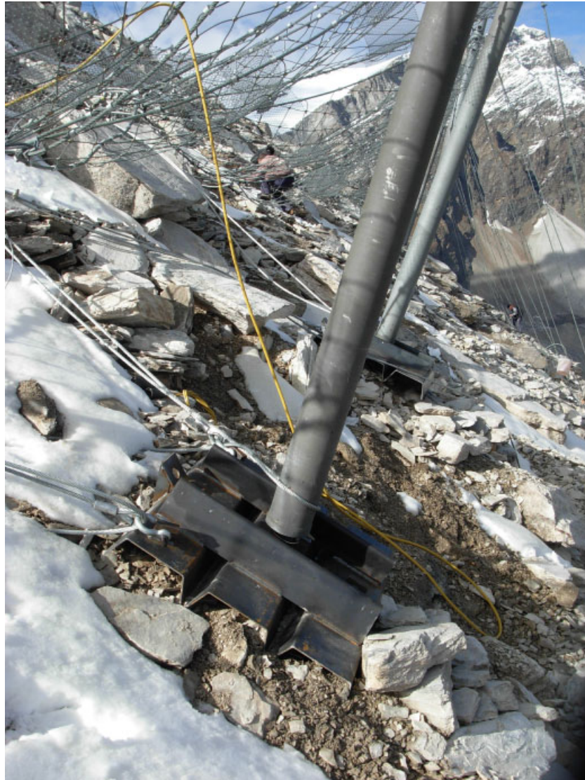
Figure 4 Floating foundation of a flexible snow net under a swivel support in strongly creeping permafrost (Photo: B. Dräyer). This figure is available in colour online at www.interscience.wiley.com/journal/ppp .
