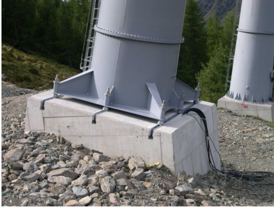
Figure 3 A laterally adjustable cableway pylon foundation for creeping permafrost terrain. This figure is available in colour online at www.interscience.wiley.com/journal/ppp .
